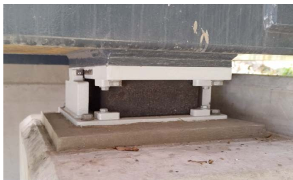
Figure 5 Proprietary designed elastomeric Type 1.2 bearing (note guide plate visible on left) underneath a steel bridge deck
